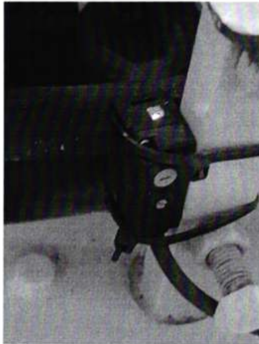
Image 3 — Photoelectric counting sensor installed on the line for unit counting
