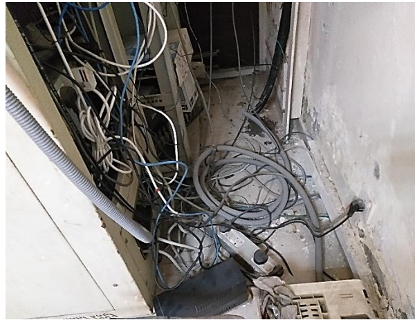
4. Loose wiring in MCC office, Peshawar
