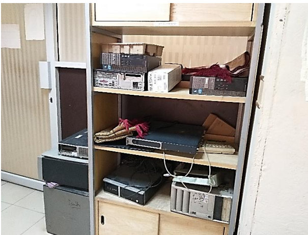
5. E-waste storage in server room, MCC office, Peshawar
