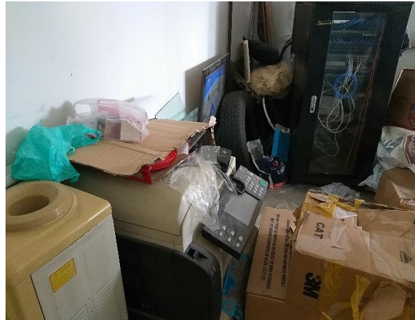
8. Storage of all types of wastes in server room, MCC office, Multan
