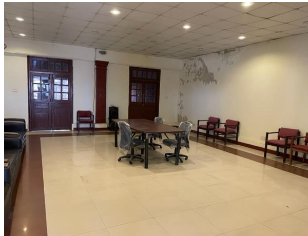
18. Infrastructure/space for installation of IT equipment at Karachi port
