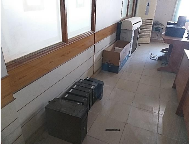
7. Inadequate storage of E-waste in open corridor, RTO, Multan
